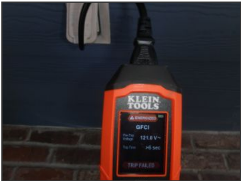
AFCI test failure--master bedroom
