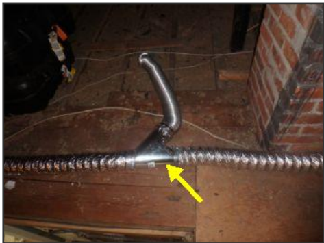
bathroom vent ducts improper tie together
