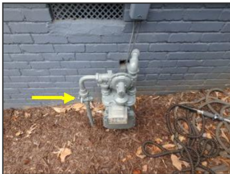
main gas fuel valve--side A
