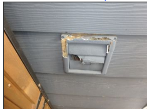
damaged weather head--side D
