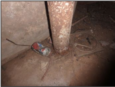
rusted steel column example
