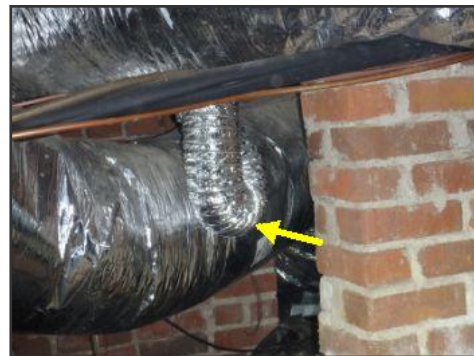
improper dryer duct material
