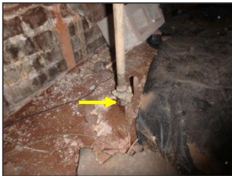
rusted and leaking main valve
