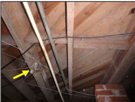
open electrical junction box
