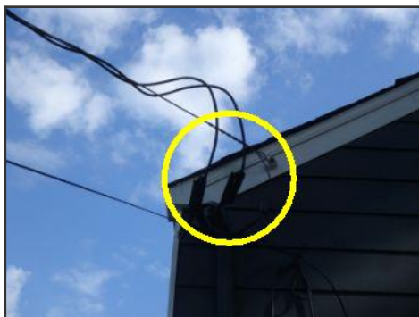
service drop connections
