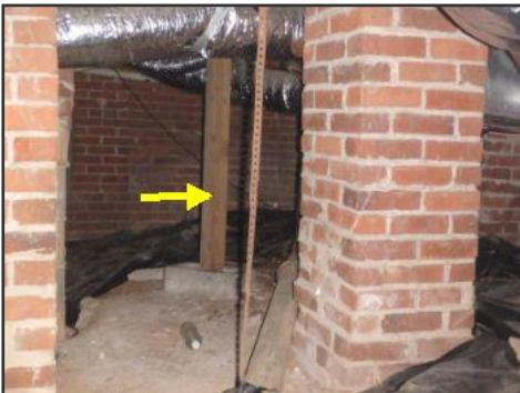
substandard floor support column
