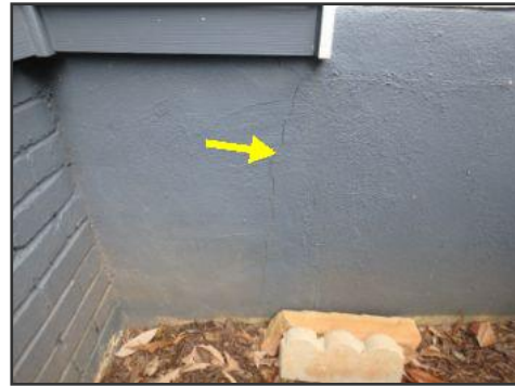
hairline crack--porch foundation
