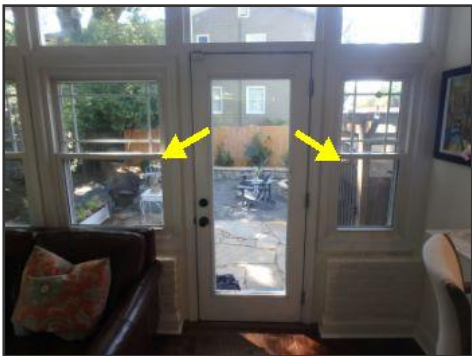
windows should have tempered glazing
