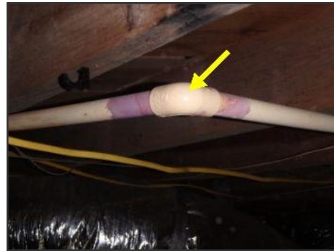
sagging pipe example
