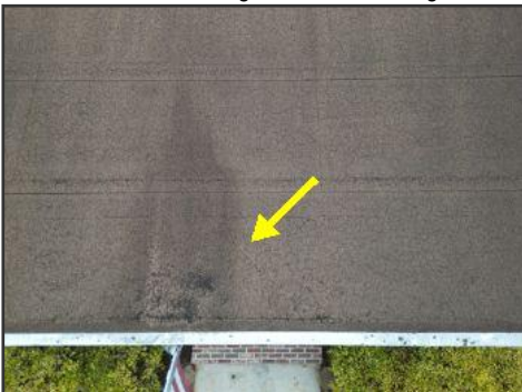
excess wear--front porch
