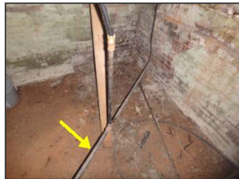
deficient support gas pipe
