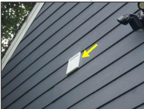
sealant needed--side B
