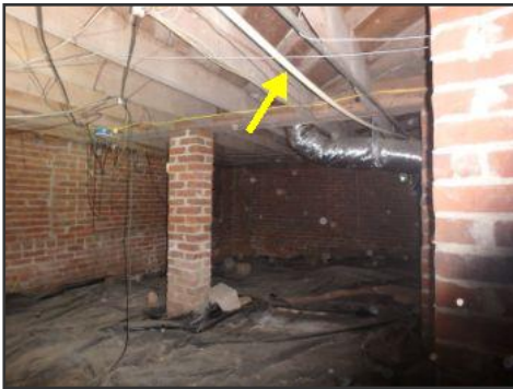
example sagging pipe
