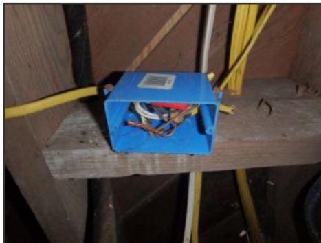
open junction box
