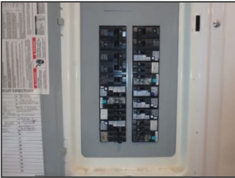
Siemens brand panelboard
