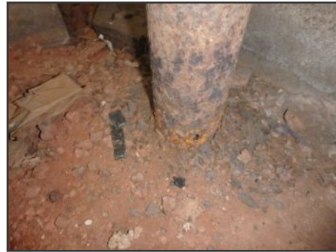
rusted steel column example
