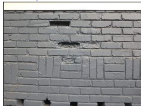
example brick spalling
