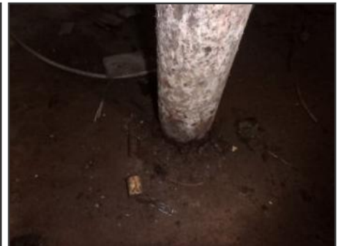
rusted steel column example
