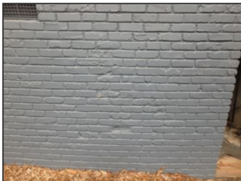
example brick spalling
