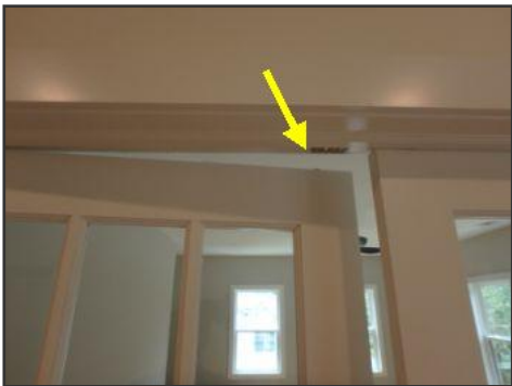
French door--deficient closure device
