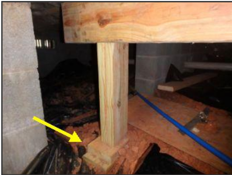
deficient girder support
