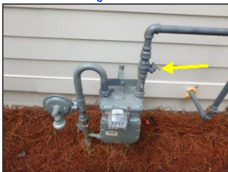
main gas valve
