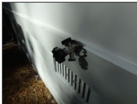
loose hose bib--side C
