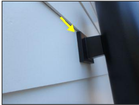
sealant needed at light fixtures' mounts
