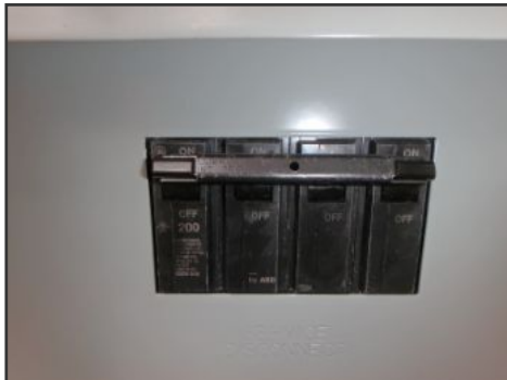
main disconnect (below meter)
