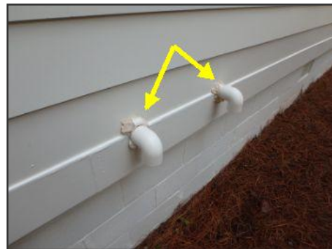
improper use of spray foam
