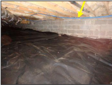
sagging water pipe
