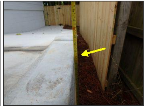
portion of driveway is over 30" from grade
