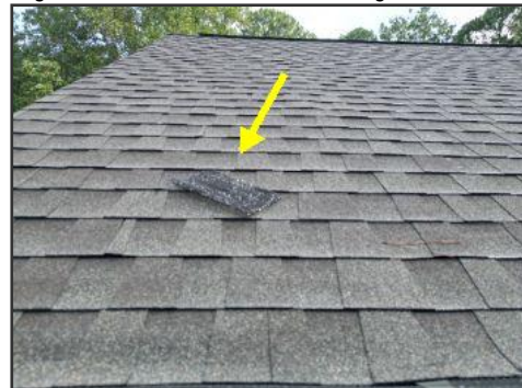
small piece of debris on roof covering
