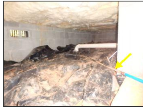
main supply line
