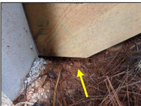
missing concrete footing under stringers
