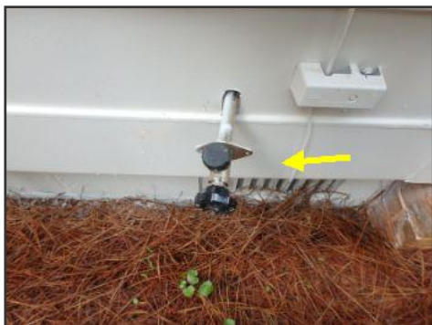
loose hose bib at side B
