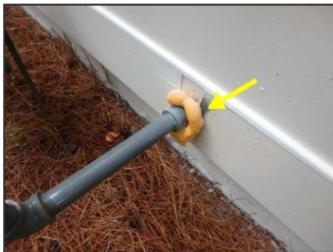
improper use of spray foam
