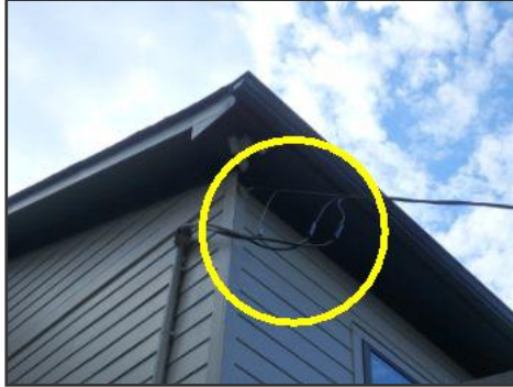
service drop connections
