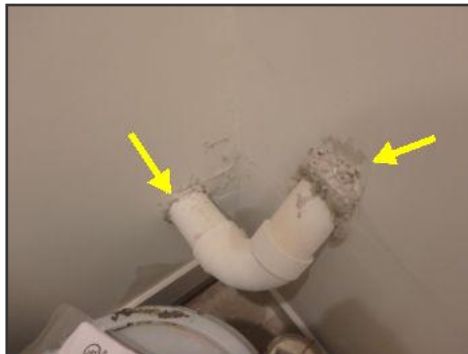
improper use of spray foam
