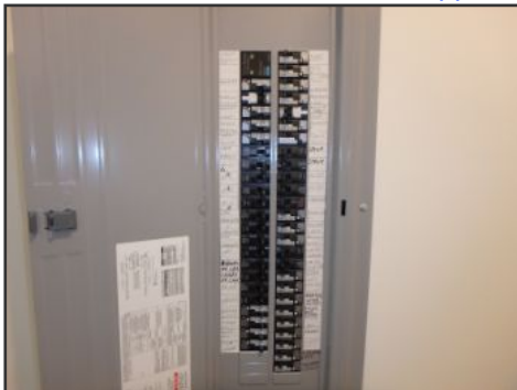
Siemens brand panelboard
