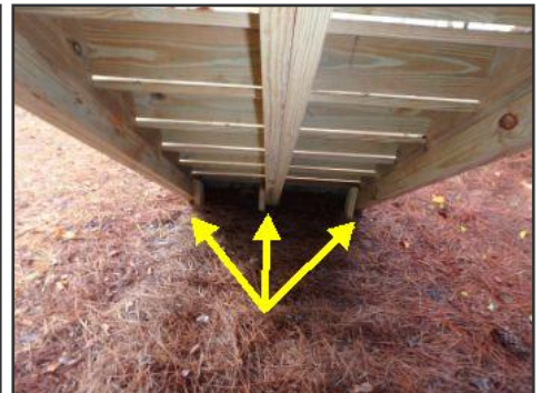
missing concrete footing under stringers
