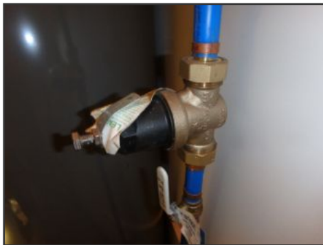
pressure reducing valve
