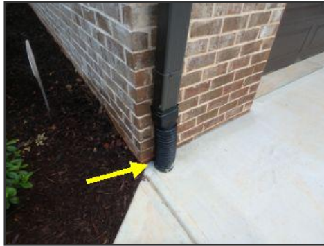
example downspout drain
